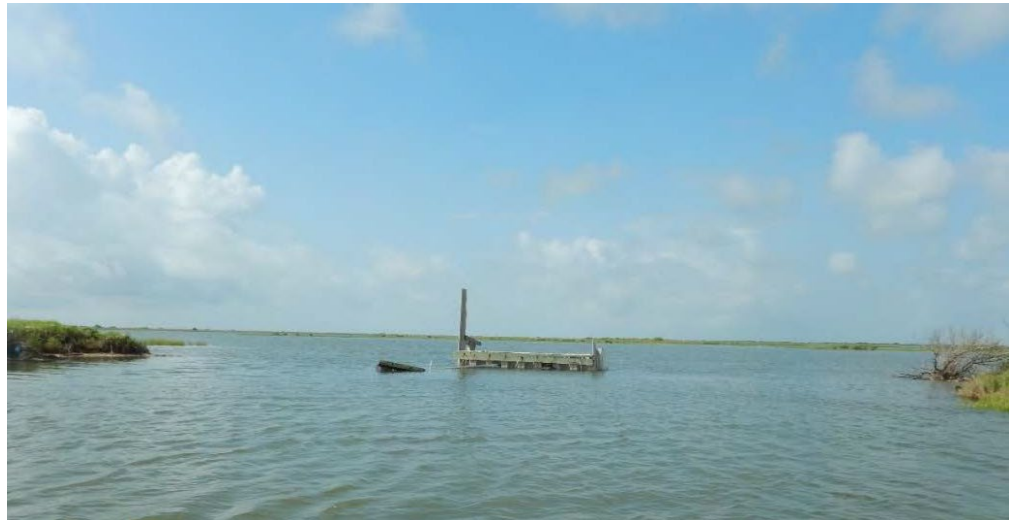
Destroyed Levee and Culvert Before Restoration
